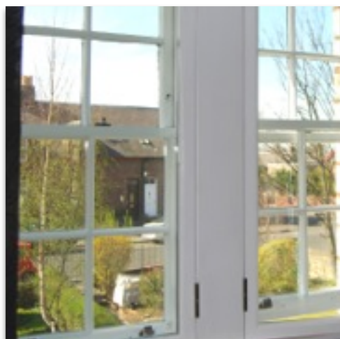
Fig. 2 Secondary glazing can be an effective way of reducing heat loss from single glazed windows
