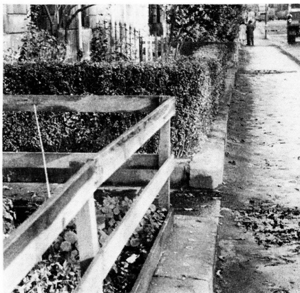
The Beaverbrook damage at the Pollockshaws Road boundary of the Conservation Area
